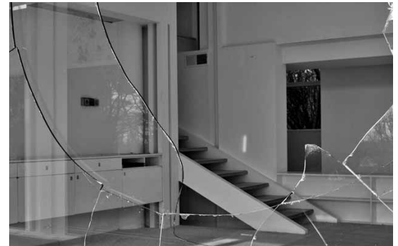
Broken window, Micheels House, Westport, CT, 2006 (photo: Chris Mottalini)
