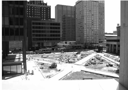
Center Plaza under construction, with Mies van der Rohe's One Charles Center on the right, April 2007. Charles Center, Baltimore, MD (photo: Olivia Klose)
