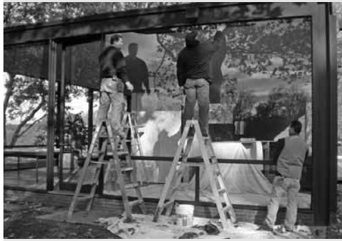
Replacing the damaged pane at Johnson's Glass House. The Glass House, New Canaan, CT. (photo: Deirdre Gould)
