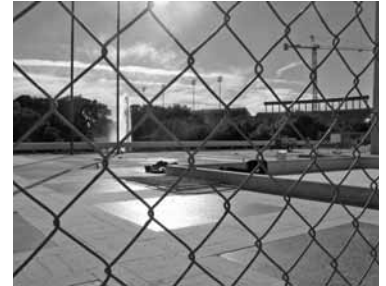
Detail of library plaza through construction. LBJ Library, Austin, TX. (photo: Catherine Gavin)
