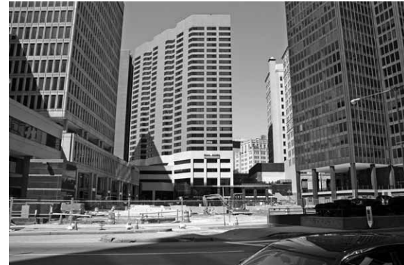
Center Plaza under construction, April 2007. Charles Center, Baltimore, MD (photo: Olivia Klose)
